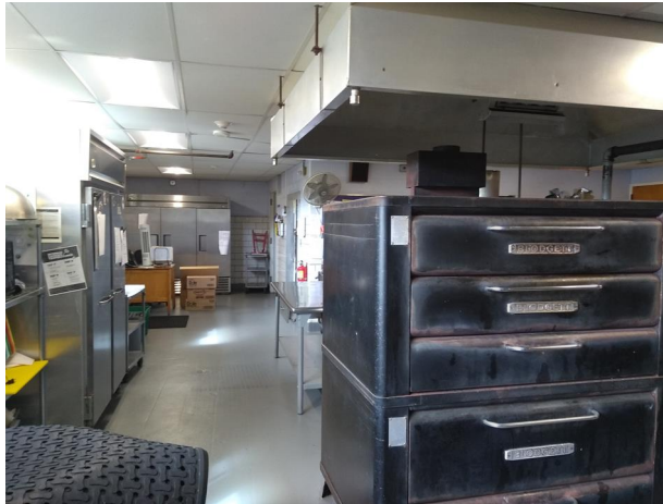
26. Kitchen equipment is very old and inefficient.
