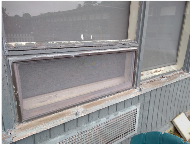
2. Original windows and trim have deteriorated.
