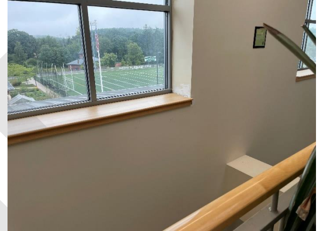
9. Several windows show signs of water damage.
