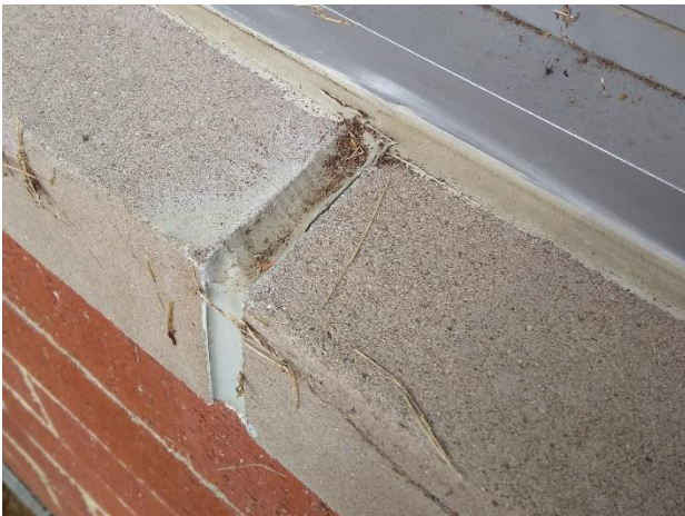
4. Some sealant shows early signs of deterioration.
