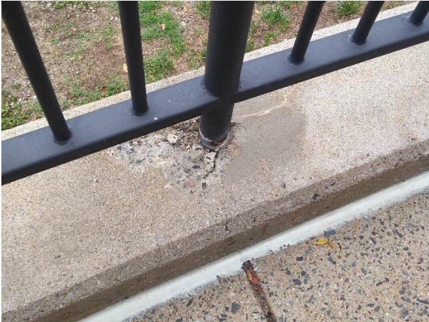
1. Concrete has spalled at some rail posts.
