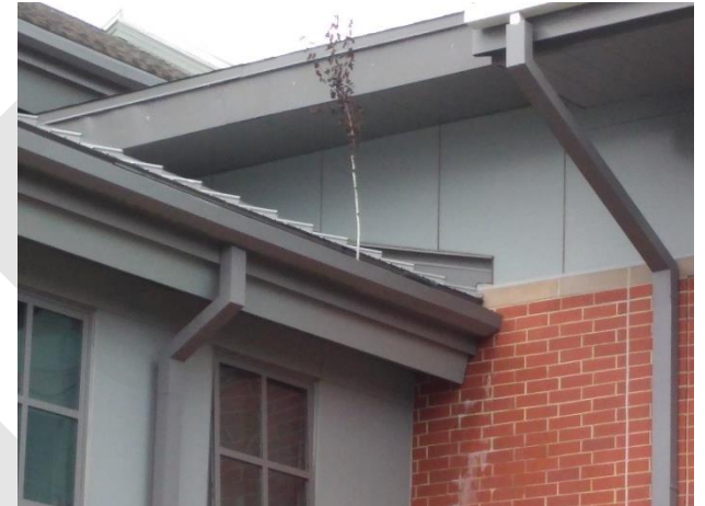
3. Some gutters are clogged with vegetation.
