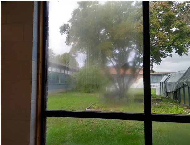
4. Thermal pane window has seal failure.
