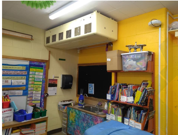
20. Classrooms have outdated and inefficient unit ventilators.
