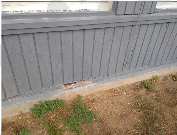
5. The wood siding is rotted and damaged.
